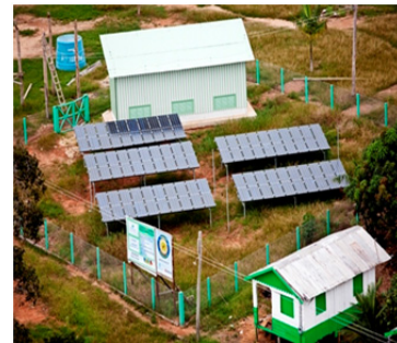
Figure 1: PV mini-grid in Amazonia. 9.6kWp for 19 Consumer Units.
